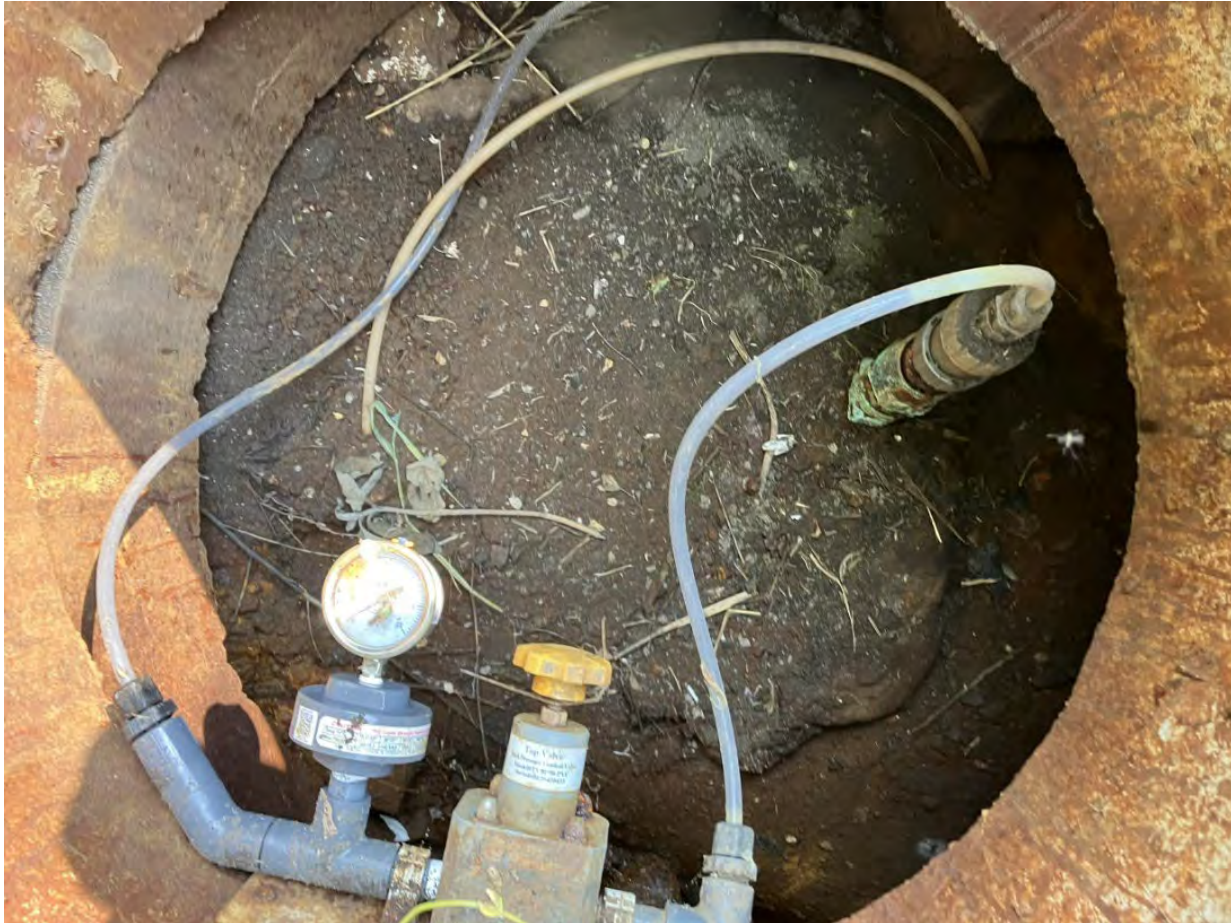
Figure 6: Interior of Chemical Feed Manhole at Injection Point.
