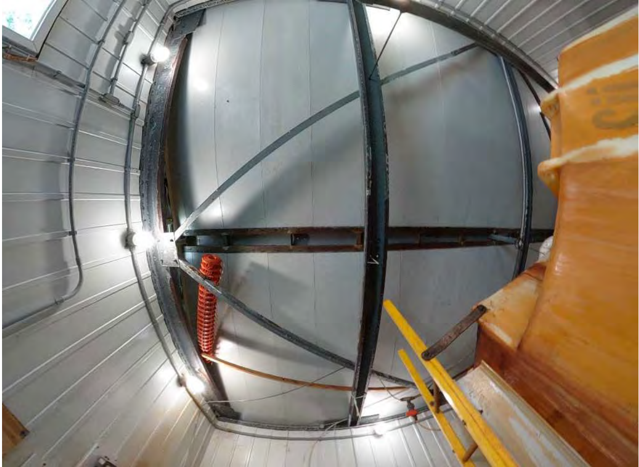
Figure 4: Interior ceiling of building showing corrosion (shape distortion from wide-angle lens).
