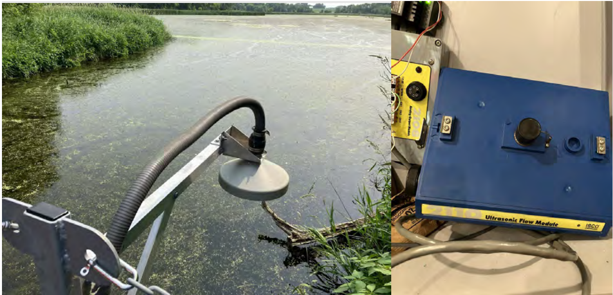
Figure 5: ISCO Ultrasonic Level Sensor and Datalogger.
