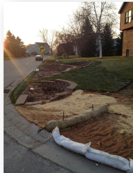
Bioretention System installed with the Clean Water Fund Grant
